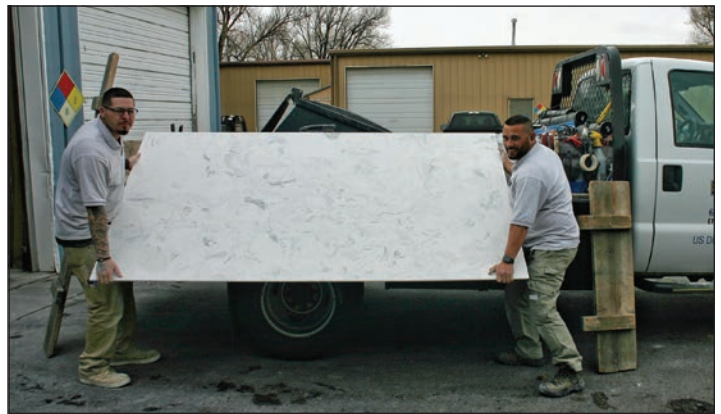
Unloading a slab from the Manstone truck are (from left): Joseph Vialpando, install helper, and Julio Lanzas, installation supervisor and lead installer.
